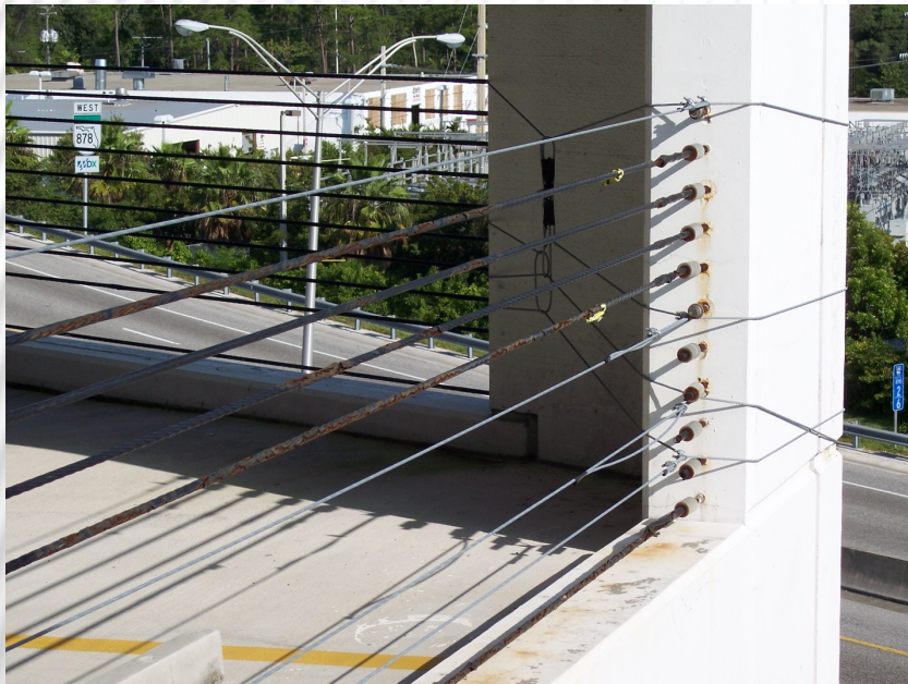
BEFORE: Badly corroded and missing cables.
